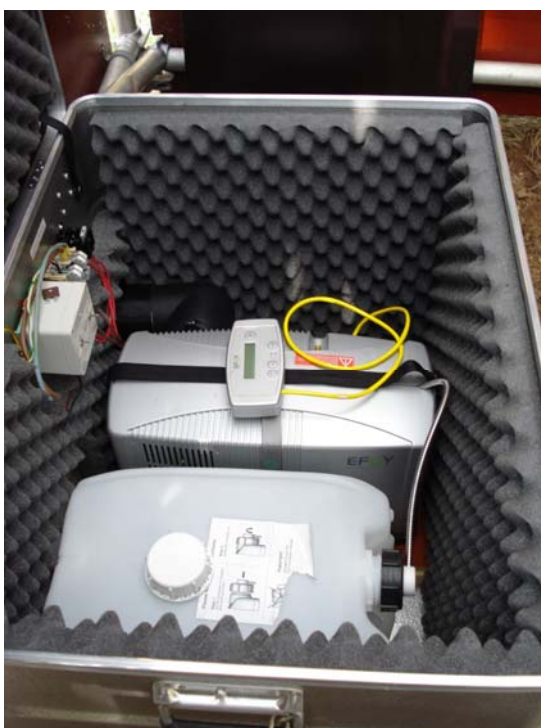
Figure 1: Direct methanol fuel cell installed at Loobos site
