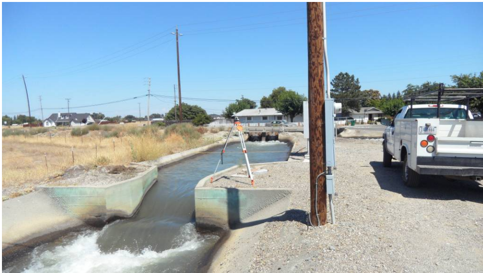
Figure 55. Example of a poor installation site: upstream is a control gate; downstream is a drop in elevation with turbulent flow
